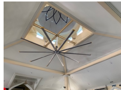
Figure 1: High-volume low-speed (HVLS) fan Source: Author
